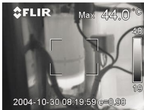
IR image shows oil and water level of compressor/ humidifier
