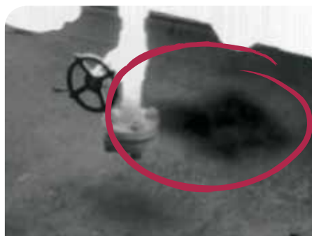
Captured gas leak from production site.
