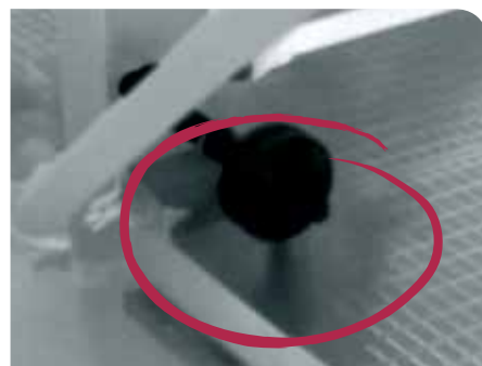
Gas leak is clearly visible on the thermal image.
