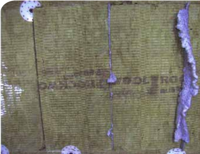
Calibration section in the insulation with open, partly filled and fully filled joint (from left)
