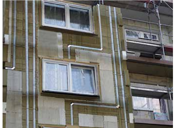
The "RetroKit" European research project: Renovation of the facade with integration of the supply and exhaust pipes in the exterior insulation (photo: Ralf H. Pelkmann).
